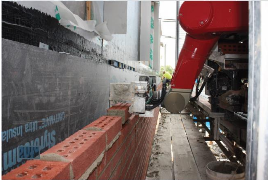
Construction Robotics SAM100 Masonry robot can lay up to 350 bricks per hour .
